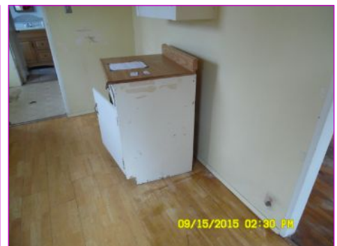
cabinet not secured to wall
