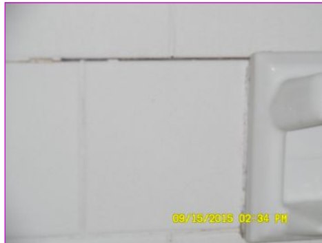
tile needs grout repair/sealing
