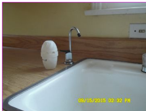
filtered water spigot not connected.
