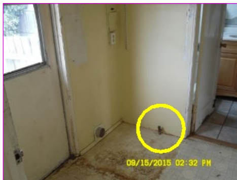
Gas line capped off. No shut off installed
