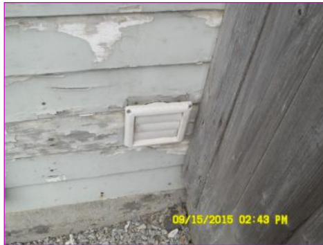
dryer vent not secured/sealed to wall
