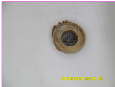
rust around drain
