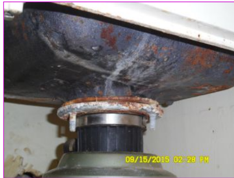
drain rusty at disposal neck.
