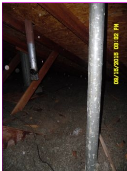
galvanized plumbing vent
