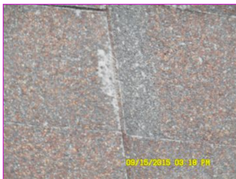
Granules wearing off on south side of roof.
