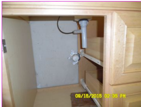
sink/faucet not completely installed
