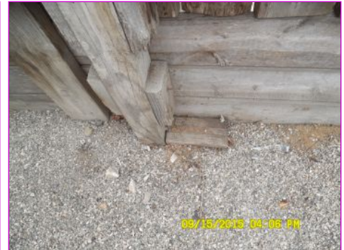
rotted fence post
