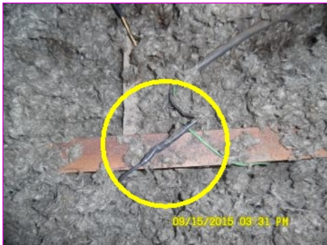
wiring junction not in box.
