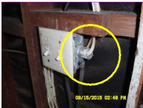
improper connection to junction box.
