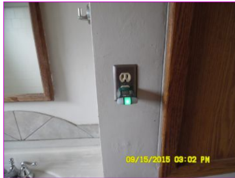
No GFI outlet in bathroom
