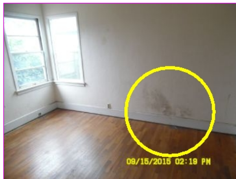
Some water stains on wall
