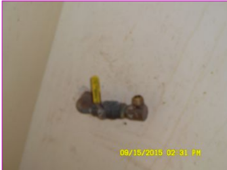
gas shut off
