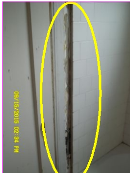
Tile edge not finished
