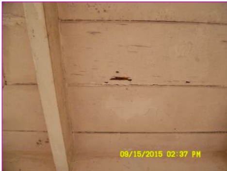
water/insect damage to wood planks
