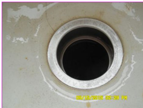
missing disposal gasket
