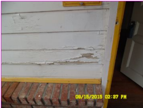
Most all of exterior needs painting.
