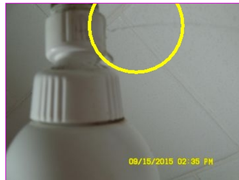
shower head connection leaks
