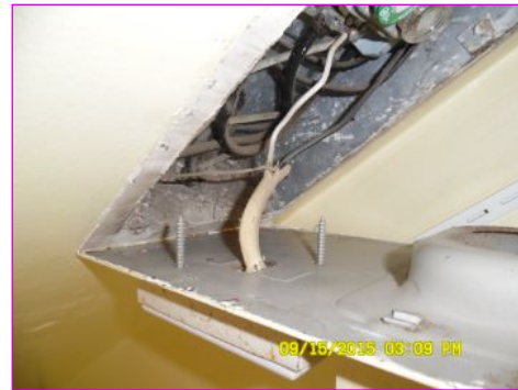
outlet installed on panel cover, not allowed and unsafe.
