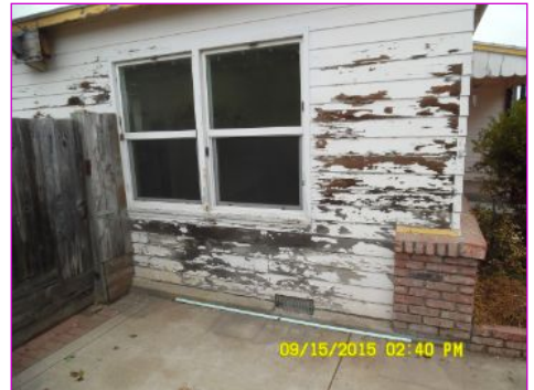
Most all of exterior needs painting
