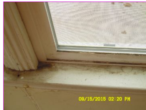
evidence of past leak at window sill
