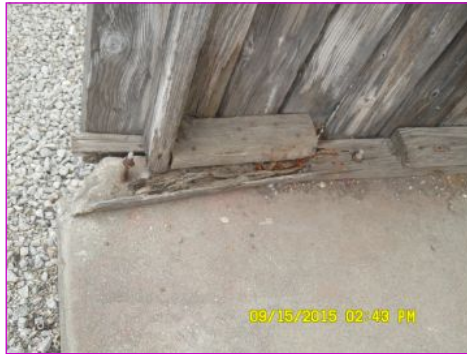
porch wood rotted.
