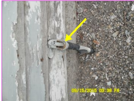
elbow needs cover.
