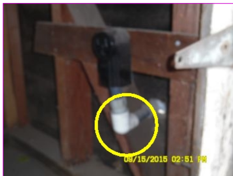
Improper pvc type for electrical
