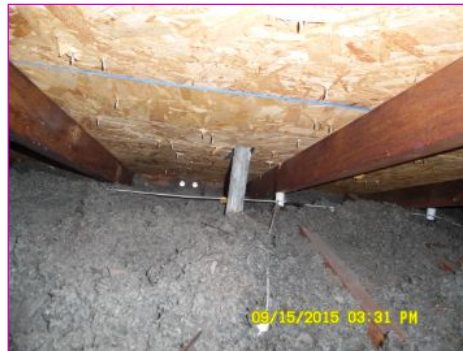
knob and tube wiring present in attic space.
