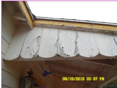
Most all of exterior needs painting
