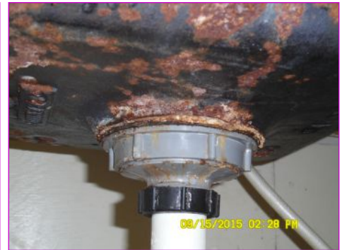
drain basket rusty.
