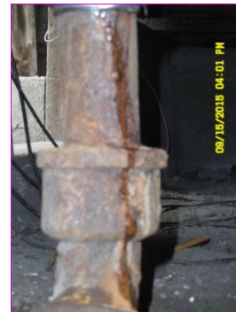
drain pipe leaking
