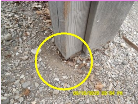
gate post rotted.
