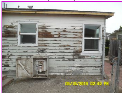
Most all of exterior needs painting
