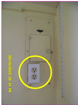
Outlet is not allowed to be installed on panel cover.
