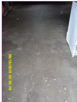
common slab crack
