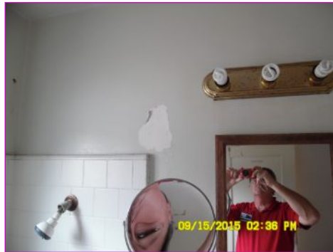
paint peeling off wall
