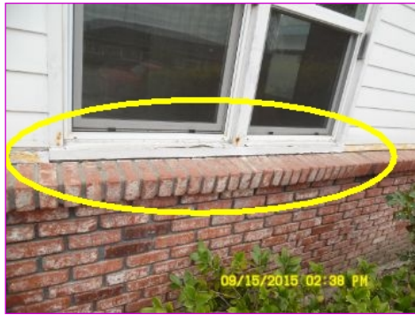
needs to be sealed up
