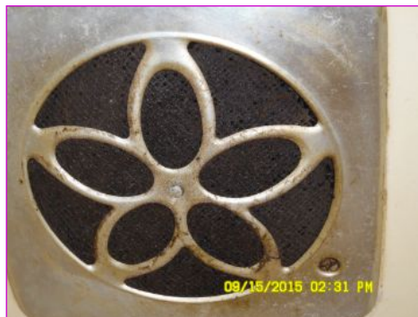
vent needs cleaning or replacement
