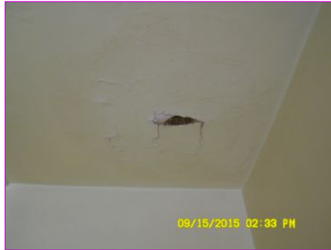
Patch of hole coming apart.
