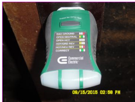
garage has grounded outlets installed but no ground found.
