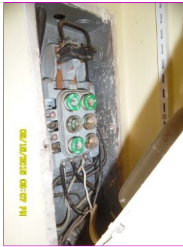
SERVICE PANEL Service Panel General Condition
