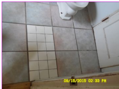
mismatched and cracked tiles
