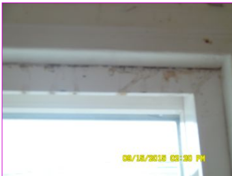
past leak at top of window
