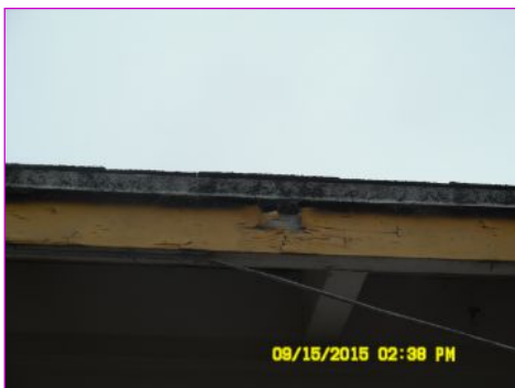
Most all of exterior needs painting
