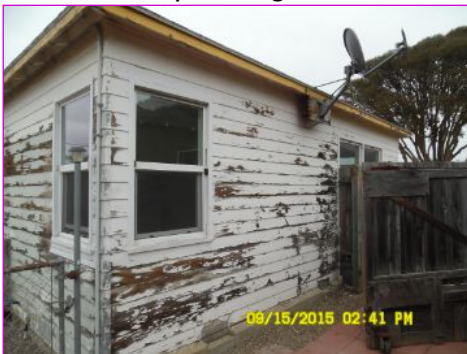
Most all of exterior needs painting
