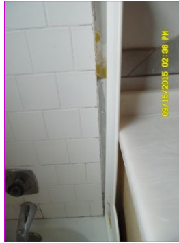
tile edge not finished
