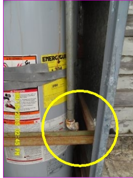
discharge pipe too high off ground.
