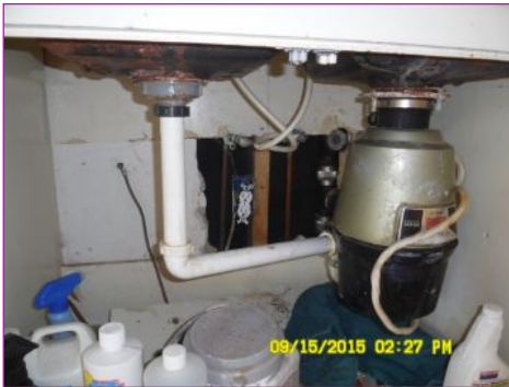
Hole in wall.
