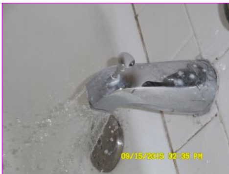
diverter does not completely seal on shower mode
