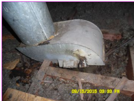
stove vent duct vent needs securing
