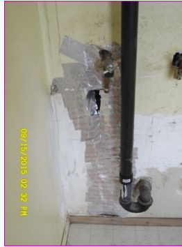
hole in wall taped up
