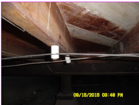
knob and tube wiring present in crawlspace.
