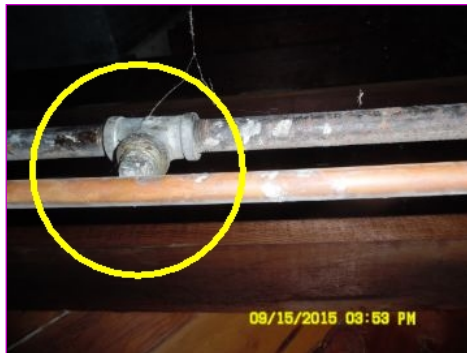
gas pipe rubbing on water pipe.
