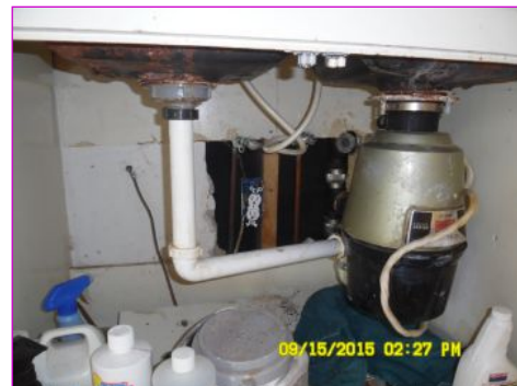
not connected to power.
