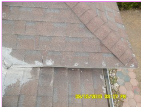
roof fasteners exposed all around roof edge.
