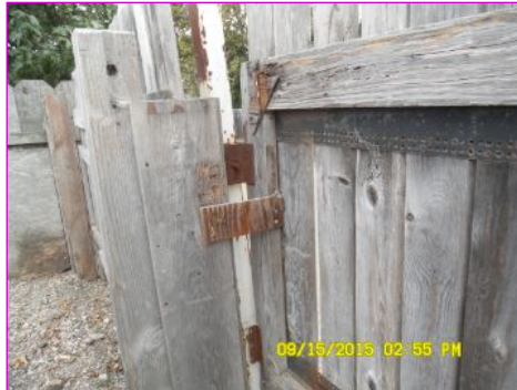
rolling gate is unprofessional installed and unsafe.
