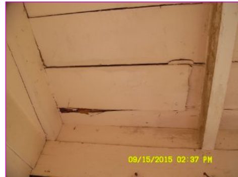
water/insect damage to wood planks
